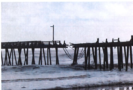
Storm damage to Capitola Wharf on Jan. 5. (Kevin Painchaud / Lookout Santa Cruz)
