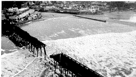
Capitola's wharf was heavily damaged in last week's storms. (Kevin Painchaud / Lookout Santa Cruz)
