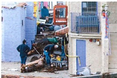
Debris litters paths between cottages at the iconic Capitola Venetian Hotel. (Kevin Painchaud / Lookout Santa Cruz)
