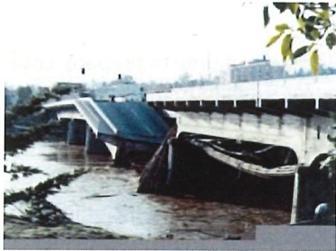
Damage from the Santa Cruz storm of 1982 (Santa Cruz County Chamber of Commerce)
