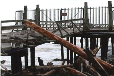
The closed and damaged pier at Seacliff State Beach in Aptos on Tuesday, January 10, 2023. (Kevin Painchaud/Lookout Santa Cruz)
